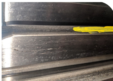
Figure 11: Example of a cracked tooth that is still intact
